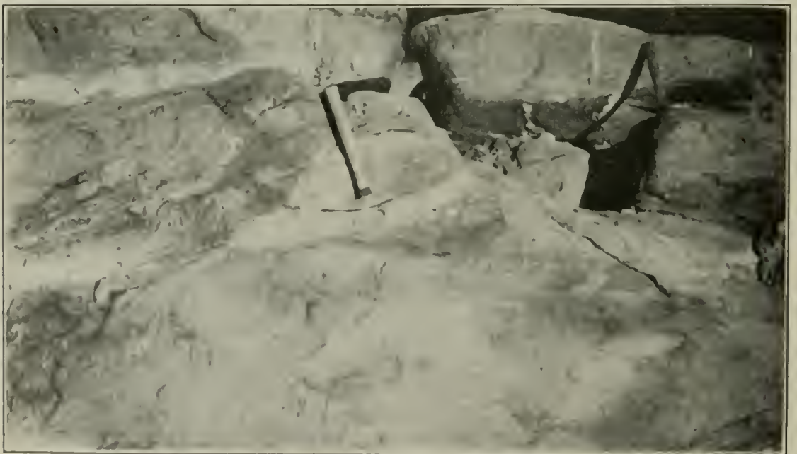
Massive amphibolite—Schistose development (at hammer). Quartz vein fillings. Characteristic Rock Formations at Dam Sites on North and South Forks of American River.
