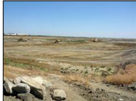
The City of Woodland has broken ground on a project that would use water from the Sacramento River as a primary supply of drinking water.
