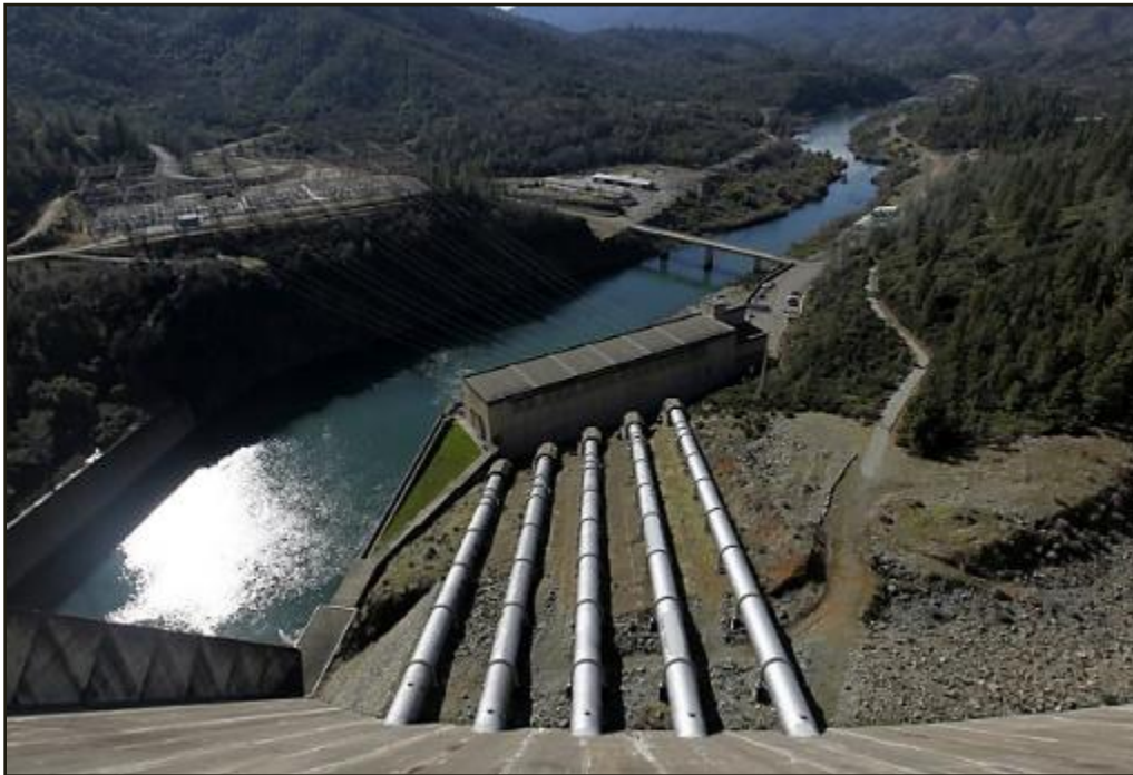
Lake Shasta water flows through five penstocks to the hydroelectric power plant at the base of Shasta Dam. A proposal to raise the dam's height drew approval in a federal report and concern in some circles. (Photo: Paul Chinn / The Chronicle)
