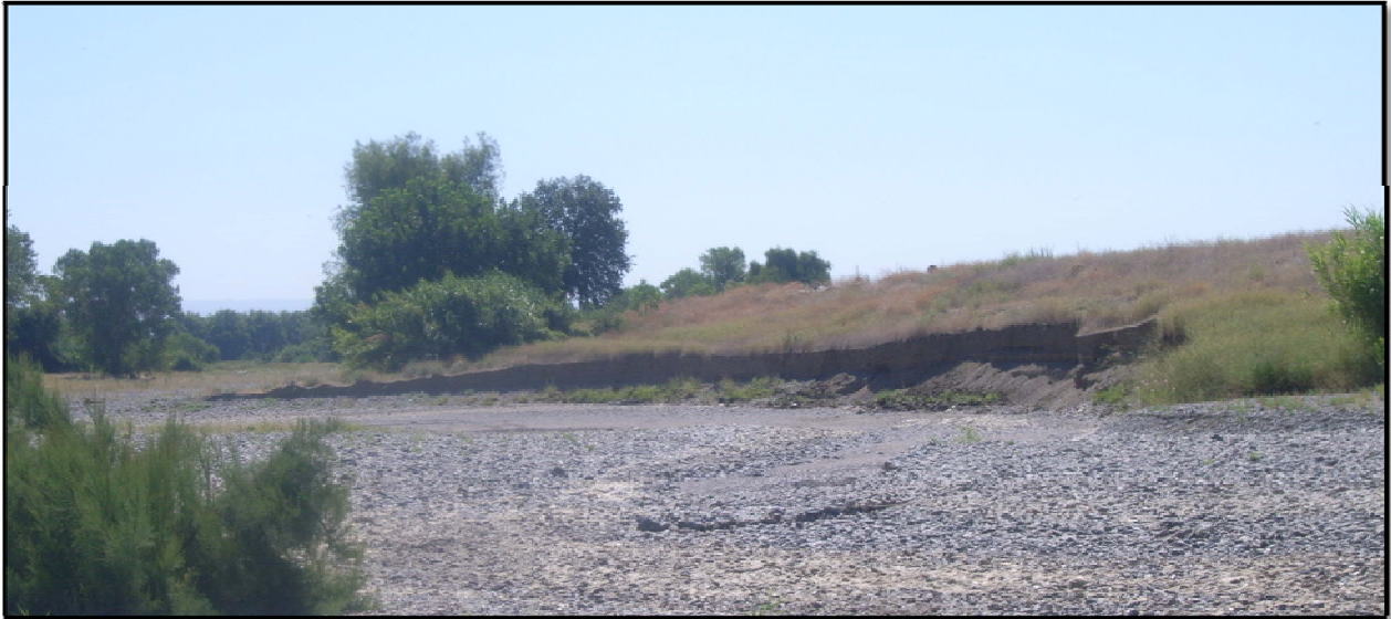
Figure 19. Typical View of the Channel and Eroding Bank of Elder Creek.
